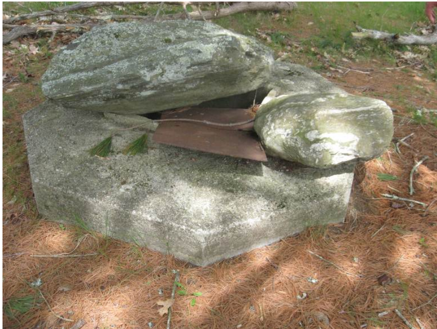
Haphazardly-placed stones and steel plate covering well near picnic shelter
