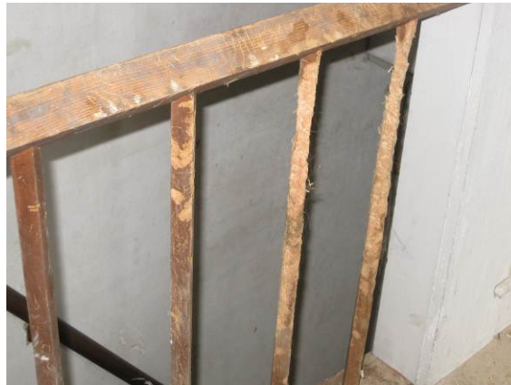
Porcupine Damage on Gardiner-Dumaesque Second-Floor Railing
